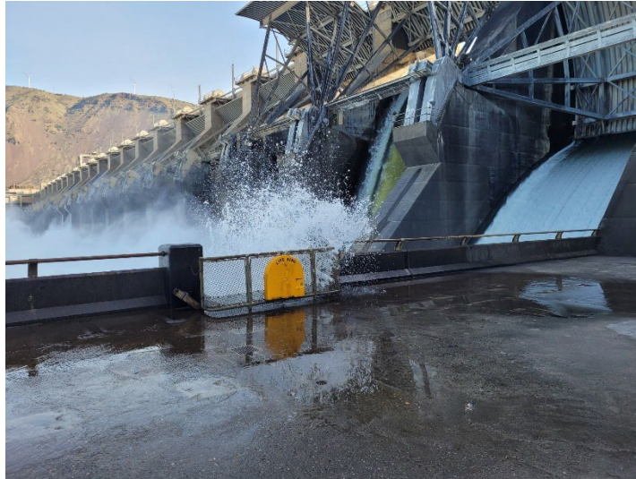
Figure 2: Image of water splashing onto the tailrace deck.
